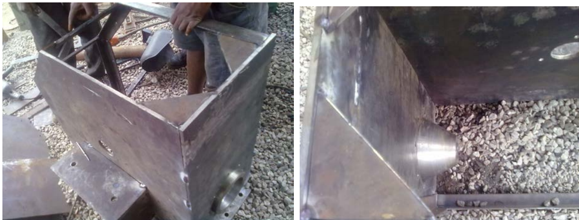
Figure 5: Turbine housing being welded together and the inside of the turbine showing the nozzle
