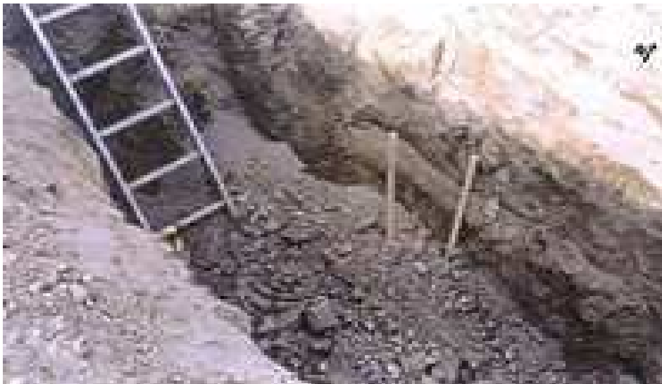
Figure 1: Excavation exercise Source: Development of Draft Construction Safety Standards for Excavations (n.d.)
