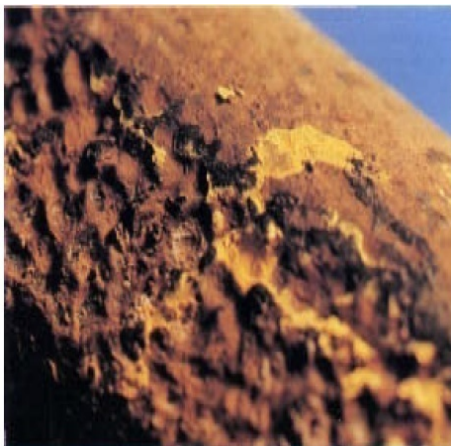
Fig-h Fly ash corrosion
