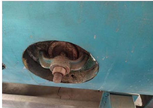
Fig-g Rusting in Manhole cover & Gasket need replacement
