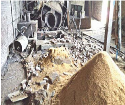
Fig-1 Boiler Accident at Jumuna Auto Rice mill, Dinajpur.
