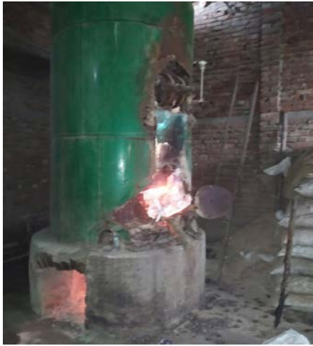
Fig-e Non standard Feed mill boiler
