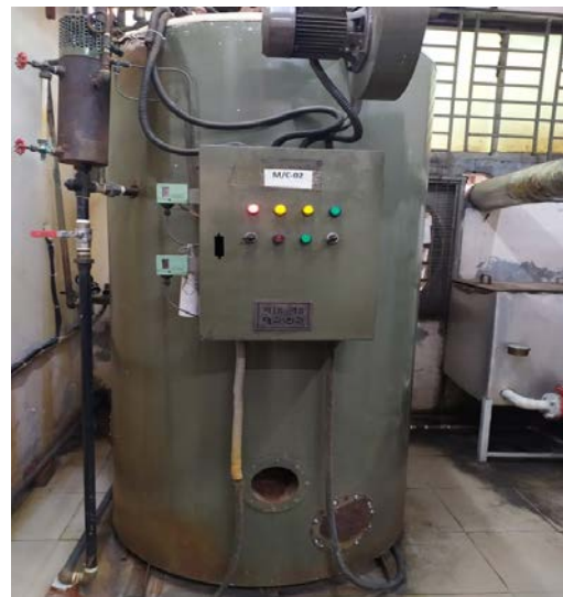
Fig-b Boiler is installed close adjacent to wall
