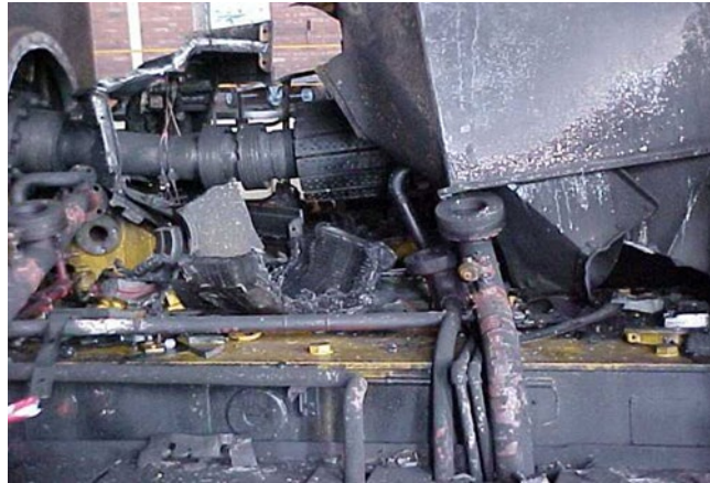
Figure 1. Steam turbine generator plant failure (Power Station Engineering Report)
