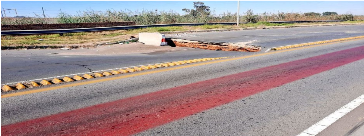
Figure 5. Klispruit Valley Road Sinkhole
