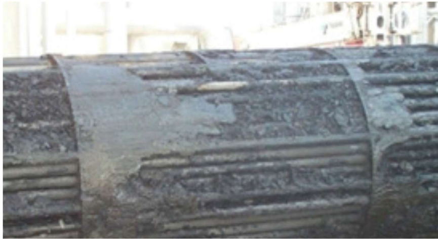
Figure 1. Snapshot of Debris on Pipe Walls of Heat Exchangers
