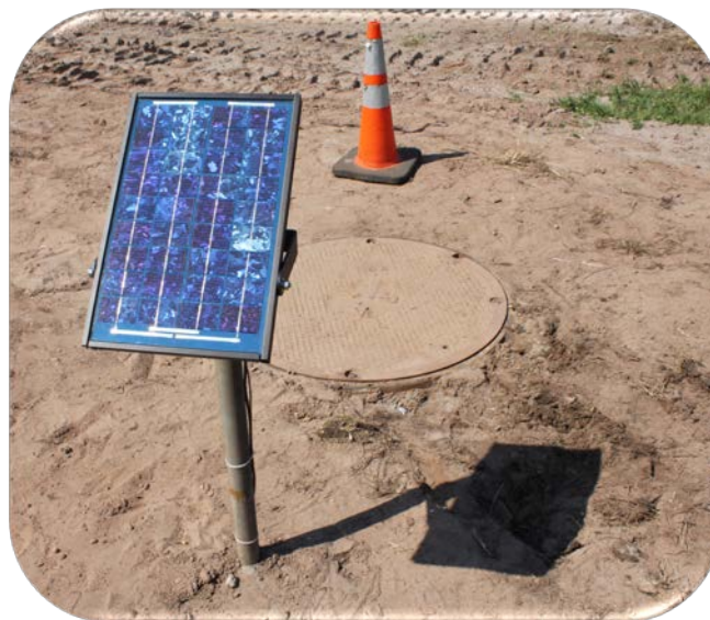
Figure 14. Close up view of small solar array for DAQ
