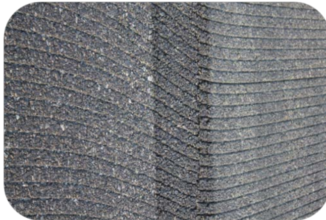
Figure 2. Example of delamination
