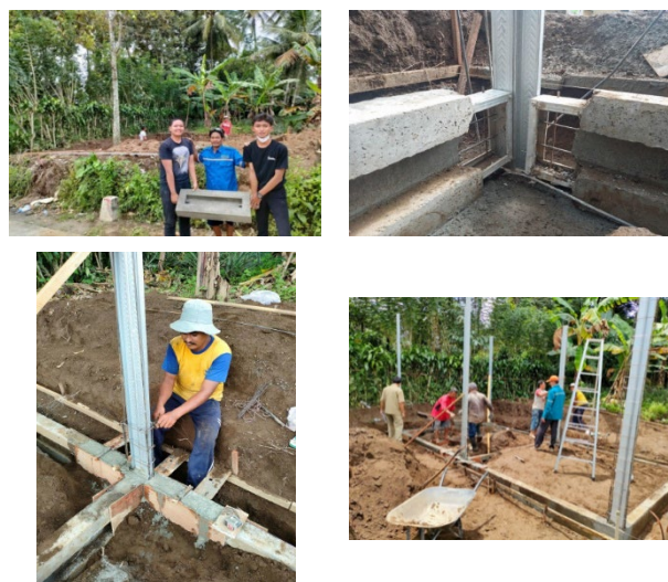
Figure 7. Implementation of composite panel houses in Semen Village, Gandusari District, Blitar City
