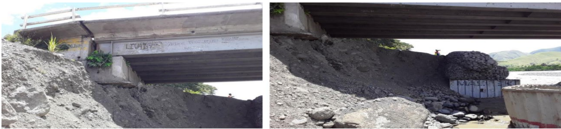
Figure 4. Hanging abutment without support (left), crumbled embankment from steady erosion (right)
