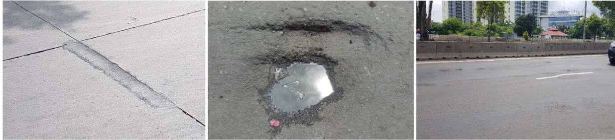
Figure 4. Identification of Road Damage on Flexible and Rigid Pavement
