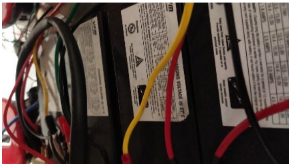
Figure 2. Four 12V, 7AH batteries powering the wheelchair
