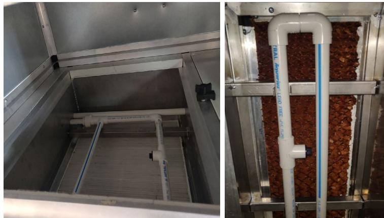
Figure 5. Heat exchangers for IDEC system
