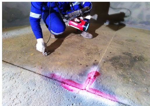
Figure 1. NDT Inspector performs thickness measurement on bottom plates and Dye penetrant test on bottom welds intersection (T welds).
