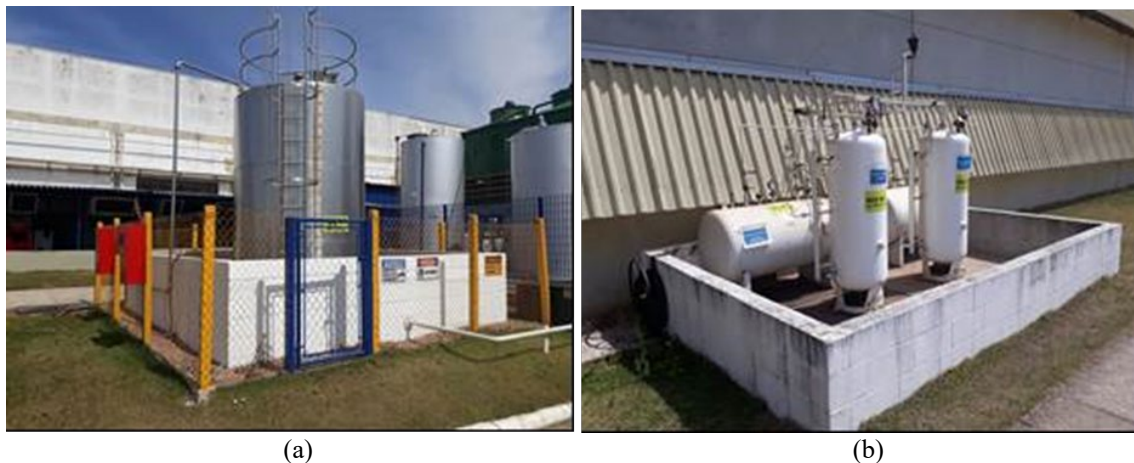
Figure 5: The images above show (a) the general methanol storage area, and (b) where the automation project will be implemented.
