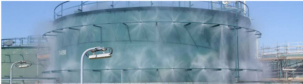
Figure 3. External Sprinkler system
