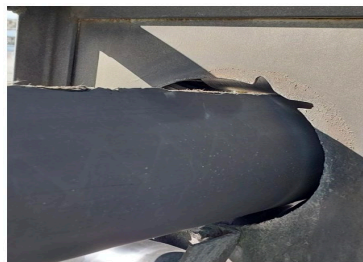
Figure 13. Belt running on sharp edge structure.
