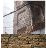
Figure 35. Damage of plaster on the southern gate (Source: author 2010)
