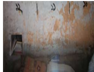
Figure 48. Excess moisture on the inside wall (Hossain 2006)
