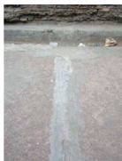
Figure 38. Major crack on floor
