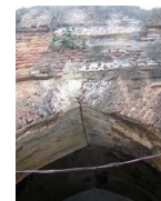
Figure 41. Crack on arch
