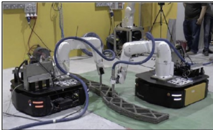
Figure 1: Robotic arm 3D printing of concrete (Prasad and Lakshmi, 2018; Rollakanti and Prasad, 2022).
