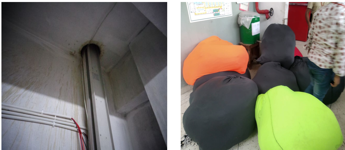
Figure 2. Unsealed (electrical riser) shafts located in the fire-rated floor/ceiling assemblies are not separated by fire-rated construction (left), Obstructed egress due to the storage of goods (right) (Accord 2021)
