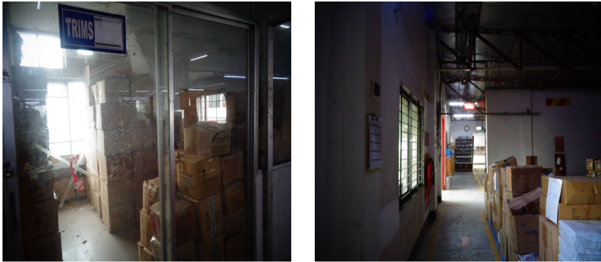
Figure 1. Areas used for combustible storage are not separated by fire-rated construction (Accord 2021)
