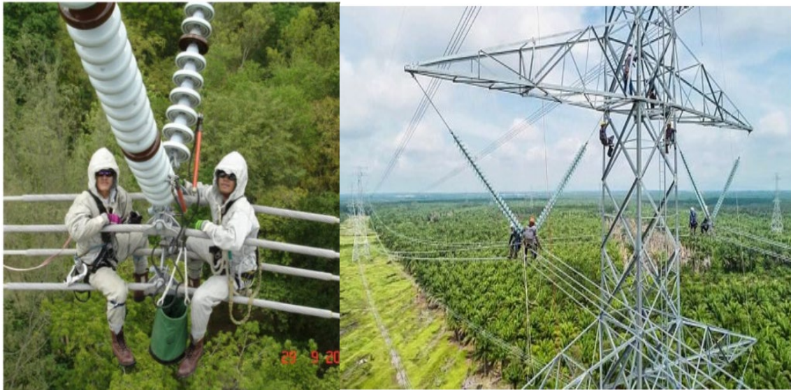
Figure 1. Characteristics of transmission line equipment repair work performed while high voltage power is turned off (Deadline Maintenance)
