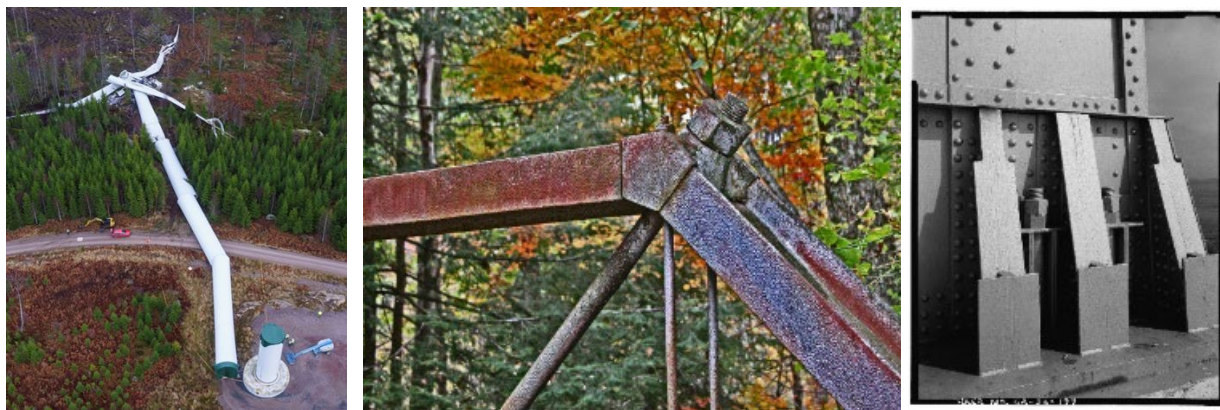
Figure 1. A wind turbine structure that collapsed due to a bolt failure (Swedish Accident Investigation Authority, 2017), picture is obtained with permission from Vestas Wind Systems A/S, Sweden (Left). Bolted bridge structure in Ohio (Center). Bolts at the base of the pier W-6 tower of the San Francisco Bay Bridge (Right). (Center and Right pictures are in the public domain, source: Wikimedia Commons).
