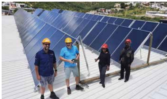
Figure 10 Partial view of the solar installation on Lady Pohamba Hospital rooftop in Windhoek, Namibia (Weiss and Spork-Dur, 2022)
