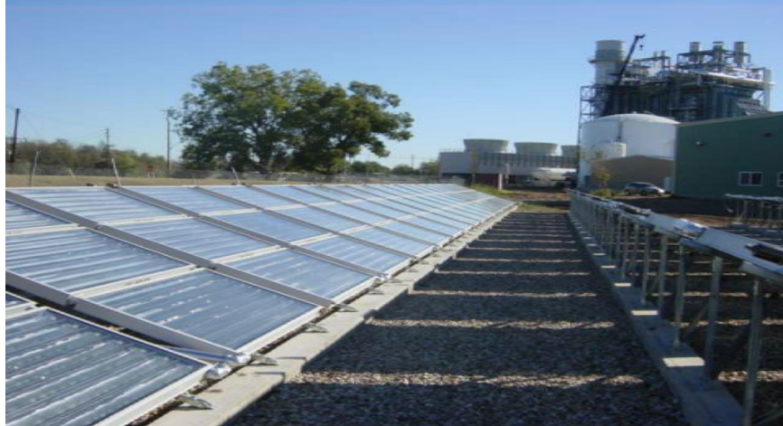
Figure 5 Arrays of solar flat plate collectors at an industrial plant in USA (Taylor, 2006)
