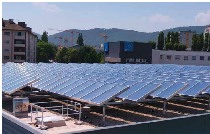
Figure 7. Roof mounted 3 500m 2 of flat plate solar collectors supply heat to drive a 660 kW absorption chiller at the company AVL in Graz, Austria (Weiss and Spork-Dur, 2022)
