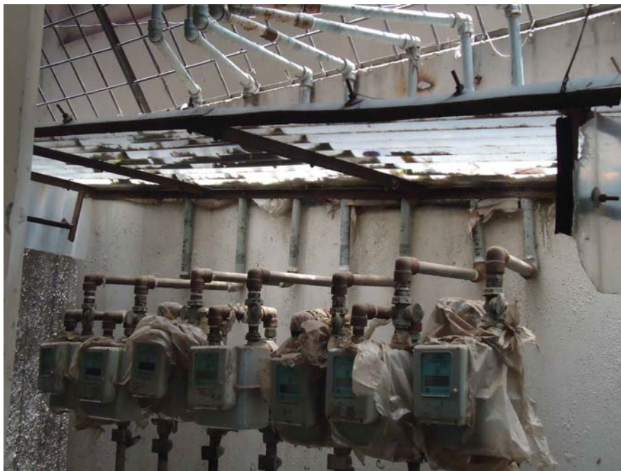
Figure 1: Previously designed prepaid gas meters installed in a house
