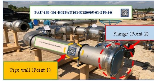
Figure 8. Mounting Location QR Code Sticker outer pipe wall
