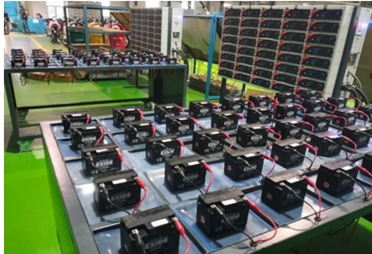
Figure 9. In-plant battery charging station with five units for enhanced battery maintenance and quality control.
