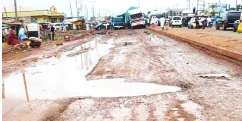
Figure 2. Bad state of Nigerian roads
