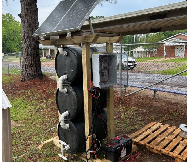
Figure 8. The irrigation system developed for this project
