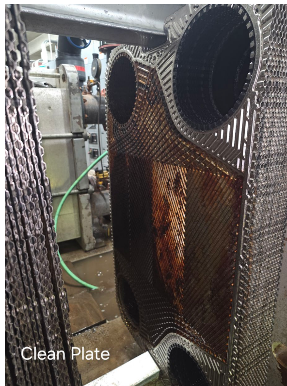
Figure 3. Photograph of heat exchanger flat plate after cleaning, which exhibits residual discoloration.
