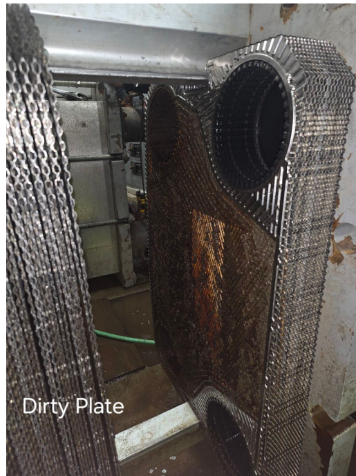
Figure 2. Photograph of heat exchanger flat plate before cleaning, with sediment fouling.
